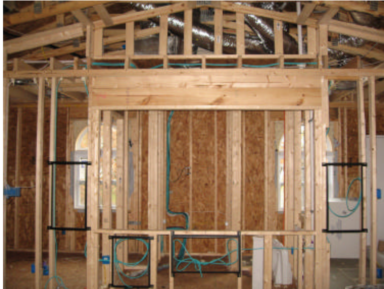
(note the proximity of in-wall black speaker frames to rough opening framing)
